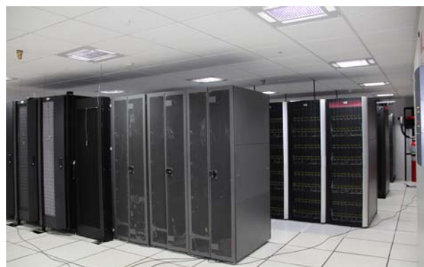
Figure 4.6 CSIR centralized 360TF High Performance Computing Facility.
