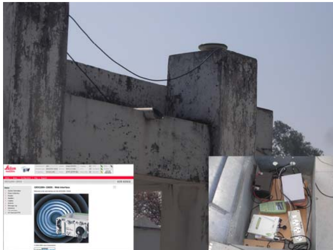
Figure 6.6 Continuous mode GPS geodetic observation facility at CSIR CBRI, Roorkee established by CSIR-4PI (ERSTWHILE C-MMACS). Insert shows (left) the web interface and (right) the instrument setup.
