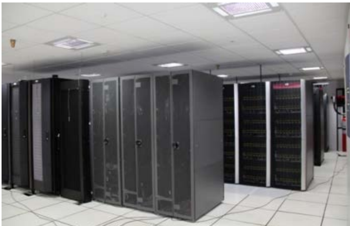
Figure 1.1: CSIR centralized 489 TF High Performance Computing (HPC) facility.
