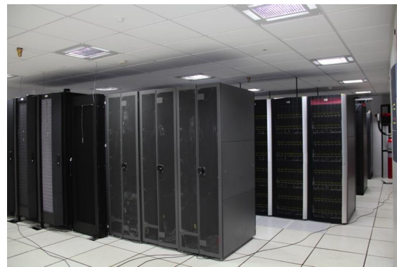
Figure 4.7 CSIR centralized 360TF High Performance Computing Facility.
