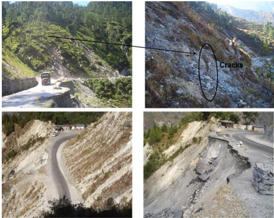
Figure 6.14 View of Landslides
